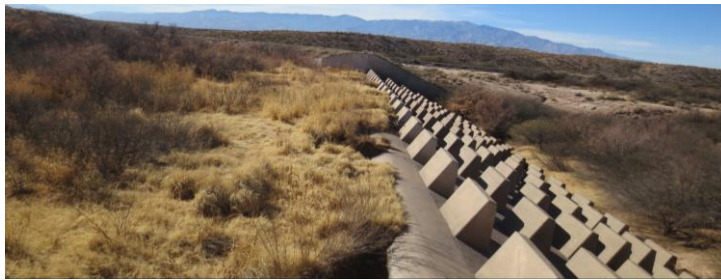
Figure 2: Overgrowth surrounding Spillway
